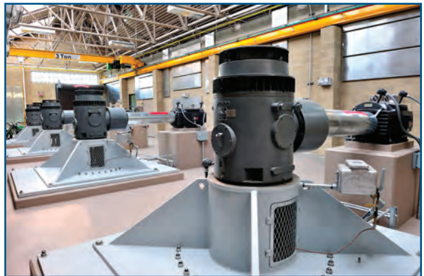
Horizontal Motor to Gear Drive
