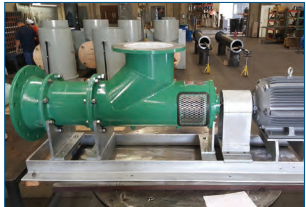
Circulation Pump at Hydraulics Laboratory
