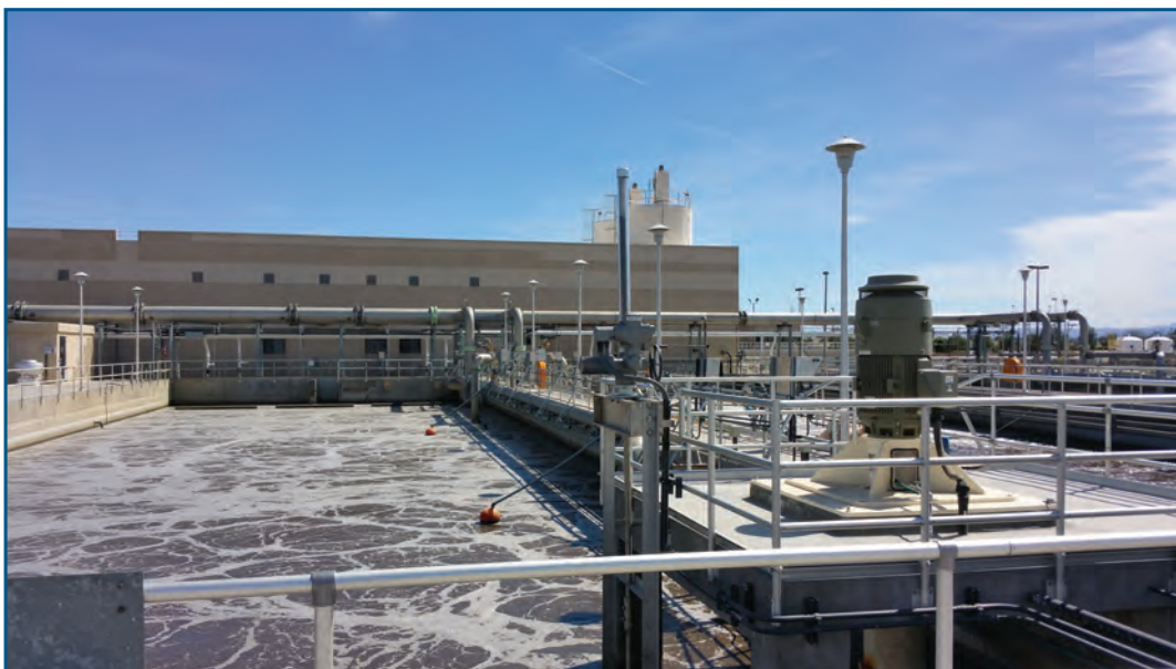
RETURN ACTIVATED SLUDGE (RAS)
