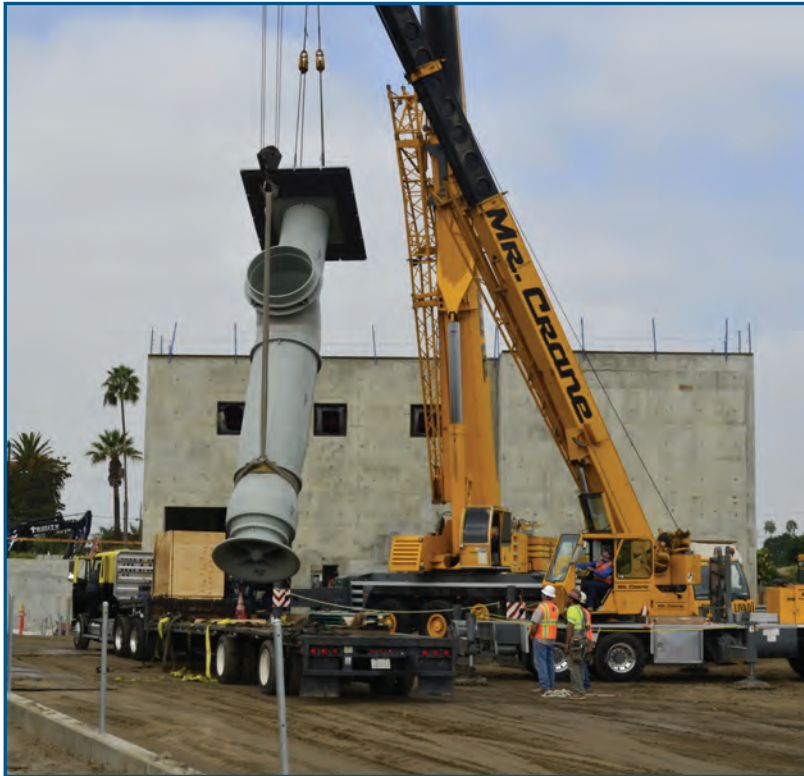
95,000 GPM STORM WATER PUMP
