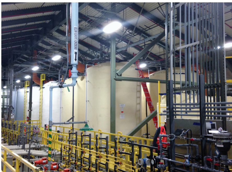
Improper installation and “hard” piping can greatly reduce useful tank life. Since polyethylene is inherently able to expand and contract, proper flexible connections accommodate this tank expansion.
